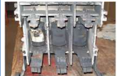
Above is a switchgear contactor after a 5 kV arc-flash event during which traditional overcurrent protection was applied. The damage required replacement of the contactor, fuse clips, copper bus, cable, control wiring, disconnect mechanism, and hardware.
