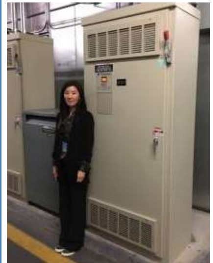
VFD Powering a 350 HP motor
