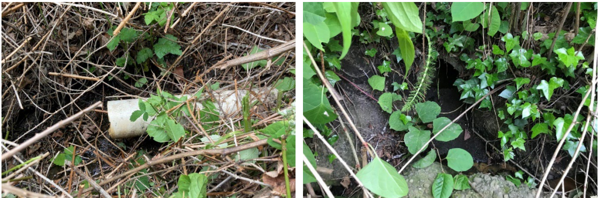
Exhibit 3-4: Views of 6-Inch-Diameter PVC Pipe Outlet into Wetland A Near Wetland Flag A14 (Left) and Approximately 10-Inch-Diameter Concrete Pipe Outlet into Wetland A Near Wetland Flag A12 (Right)
