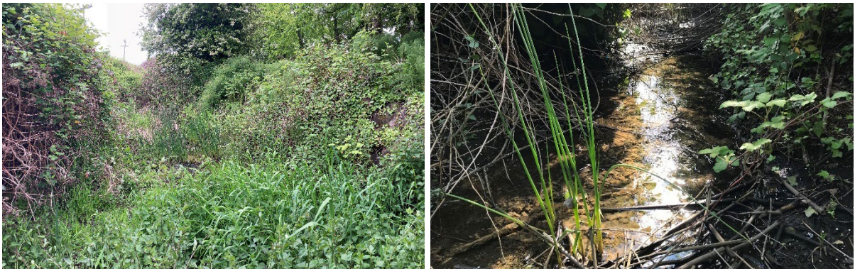
Exhibit 3-3: Views of Dense Herbaceous Vegetation and Sparsely Vegetated Areas in the West Cell of Wetland A
