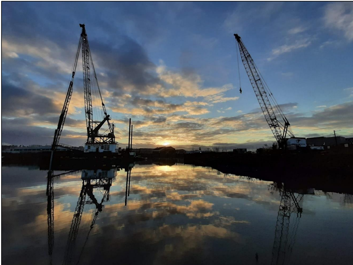
Figure 4. Cranes prepare for pile installation as morning dawns at a Duwamish River restoration site. Credit: Sasha Ertl/Grette Associates
