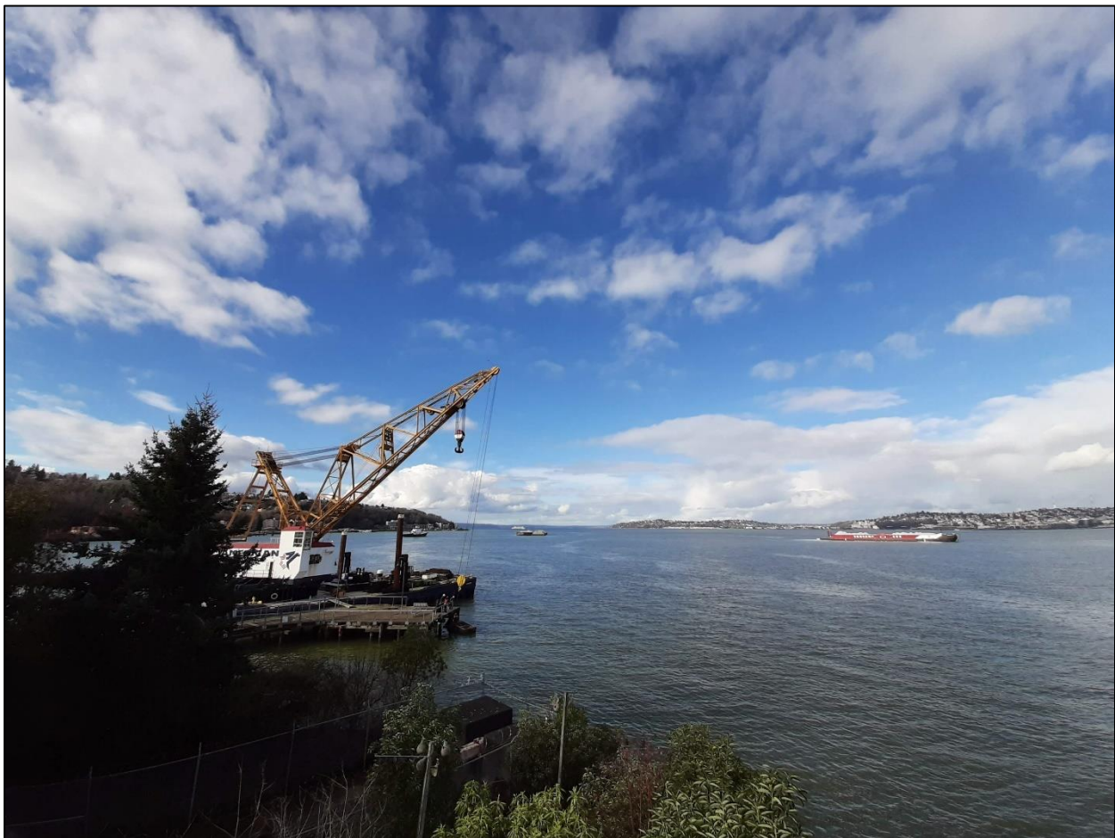
Figure 3. A crane prepares for vibratory pile driving as various vessels maneuver throughout Elliott Bay. Credit: Sasha Ertl/Grette Associates
