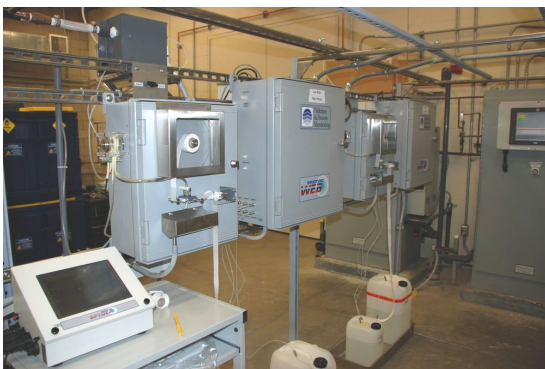
Water Testing Equipment
