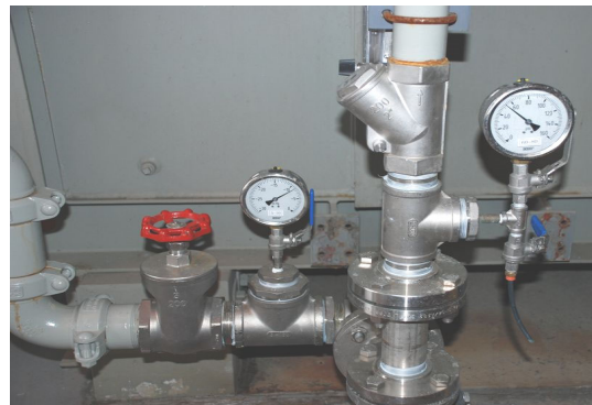
Valves and Gauges
