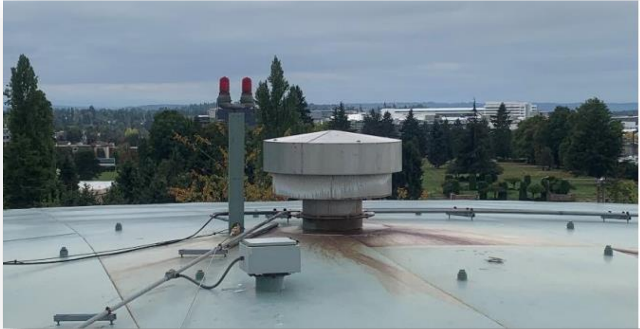
Cap Vent Moderate rust needs removal
