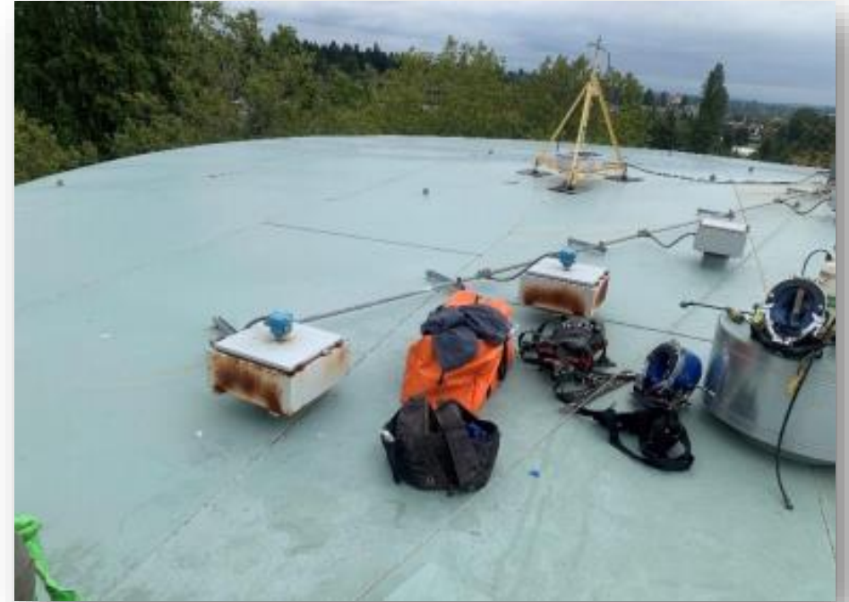
Telemetry boxes Deteriorated coating
