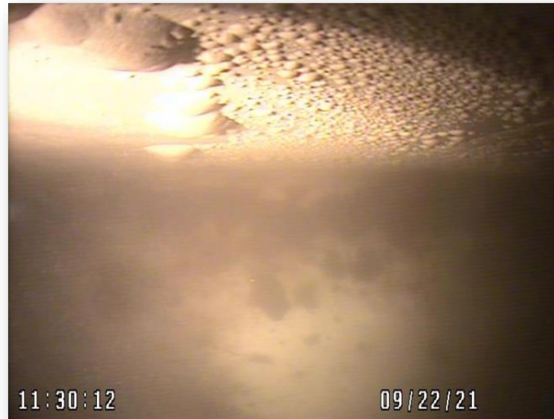
Bubbling/failing of interior coating
