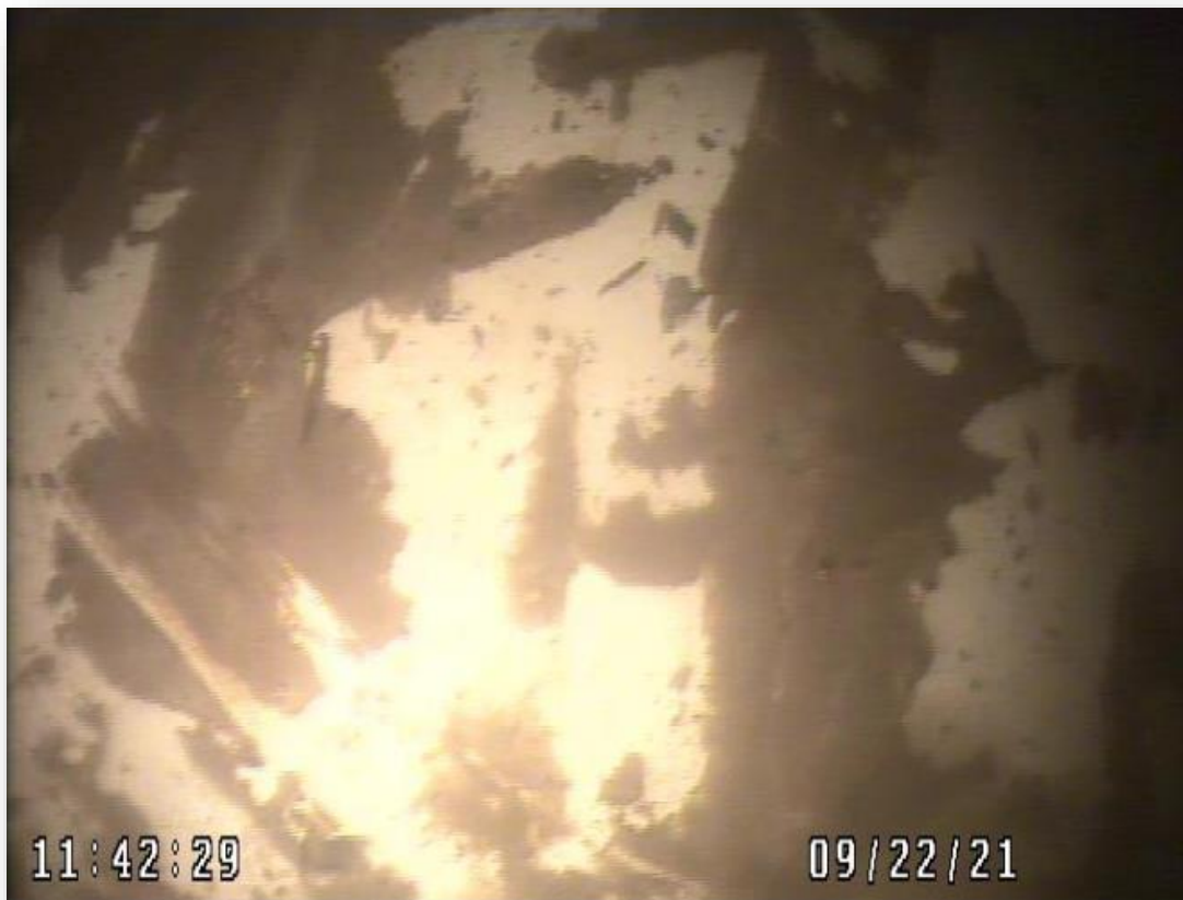
Significant rust on interior tank surfaces
